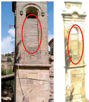
Figure 16: Documentation of anthropogenic change of the bell tower at the church of Saint Kirikos and Ioulitis. In circle the recent intervention in the church (photo in the left / 3D laser scan model in the right)
