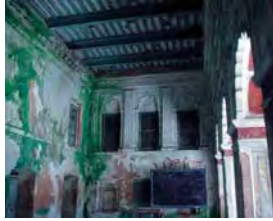
Figure 18: Damp in Wall
