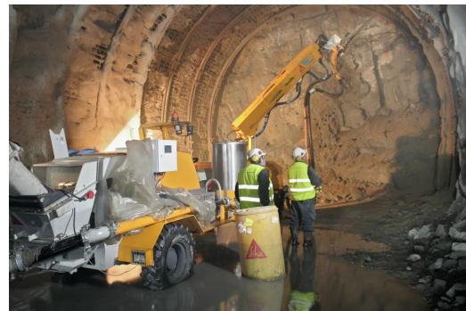
Figure 1: Concrete spraying system.
