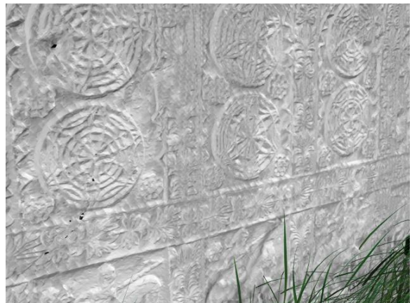
Figure 7. Incorrect orientation, 15:00 –close up
