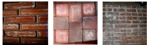
Figure 1: Walls affected by efflorescence
